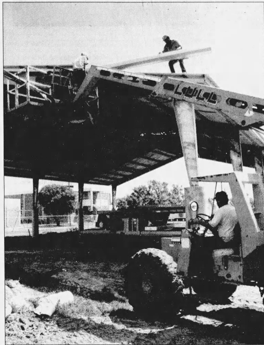
Construction workers finish the roof of the Yeager Elementary School playground pavilion. Completion of other pavilions is on hold because of a dispute between CCISD and the contractors. George Gongora/Caller-Times
