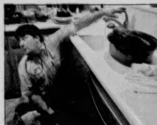
Sacramento Bee/Letzie Sterling Roto-Rooter's James Kellerman unclogs a drain at Donna and Jeff Garcia's home Friday, the busiest day of the year for plumbers.
