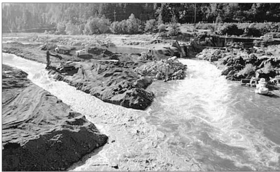
Two channels of the Rogue River in southwest Oregon meet Friday after two berms were removed from the north side, on left, allowing free flow for first time in 88 years.
