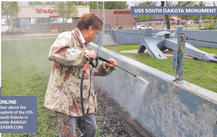
Robert Ruf is part of an effort to polish up the USS South Dakota monument at Sherman Park in Sioux Falls. The monument will be sandblasted and power washed and concrete repainted before a June 27-29 reunion of U.S. Navy veterans. JON WALKER / ARGUS LEADER
