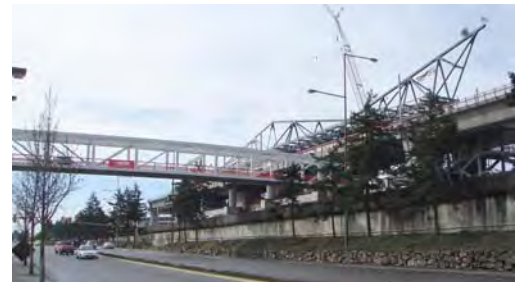
Sound Transit Light Rail Line – Airport Light Rail Station under Construction. Pedestrian bridge was recently installed.
