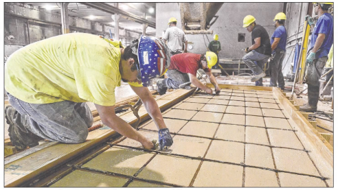
Kenny Manz wires together pieces of rebar while pouring precast concrete wall sections Friday at Gage Brothers in Sioux Falls. ELSHA PAGE / ARGUS LEADER
