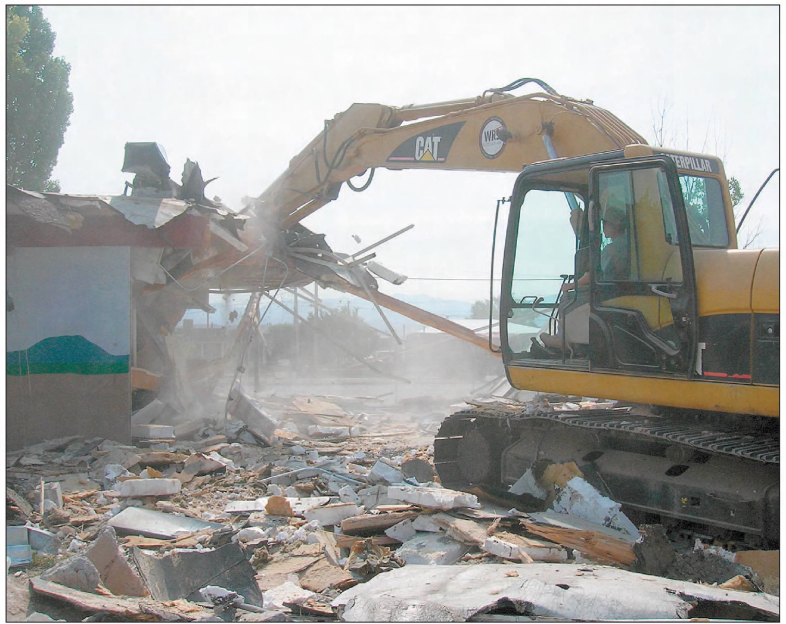
Workers from Leroy's Excavating, a subcontractor for Blue Sky Builders, tear apart a wall at Española Elementary building. Demolition began Tuesday, and Española Superintendent David Cockerham said an addition to the school will open on time for the upcoming school year. Plans call for additional classrooms and new administrative offices.
