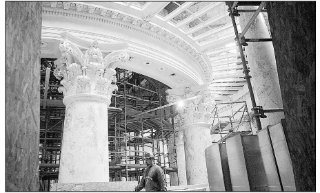
The Capitol restoration and expansion project is on schedule, but has had to revise its budget. Above is a view from the fourth floor looking back at the rotunda.
